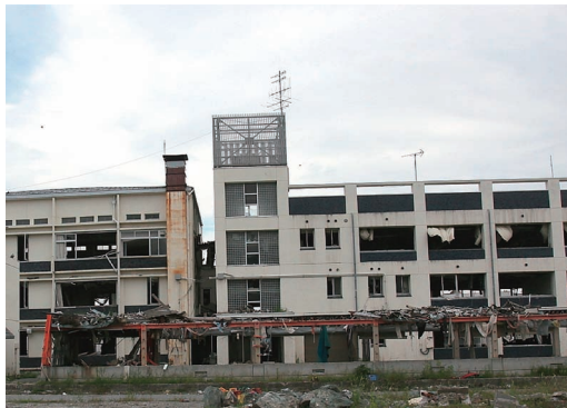
Fig. 1. City hall destroyed by Tsunami up to 3 rd floor (Rikuzentakata).
