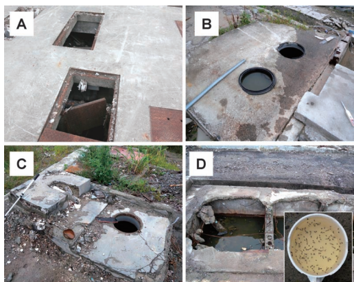
Fig. 2. Septic chambers and related structure with mosquito larvae scattered in the Tsunami affected areas.
